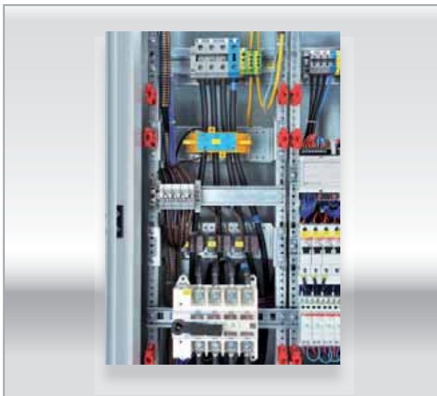
Residual and operating current monitoring in the incoming feeder
