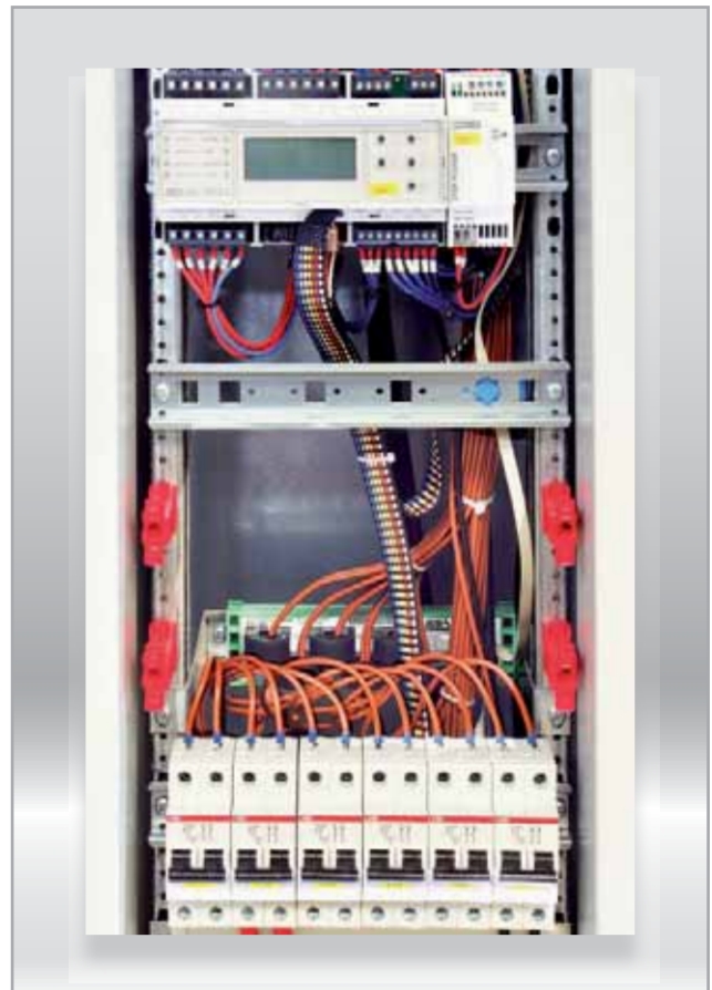
Detail of an IT system distribution IPS-ICU-710 with Insulation fault detection system ( IFS )
